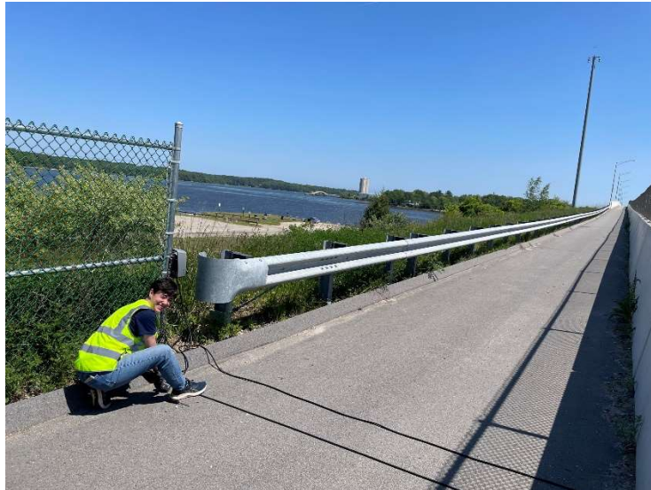
FIGURE 5 - 2023 SUMMER INTERN TROY IS SEEN INSTALLING TUBING FOR THE CYCLIST COUNT ON THE LITTLE BAY BRIDGE IN JUNE 2023. SOURCE: SRPC 2023.
